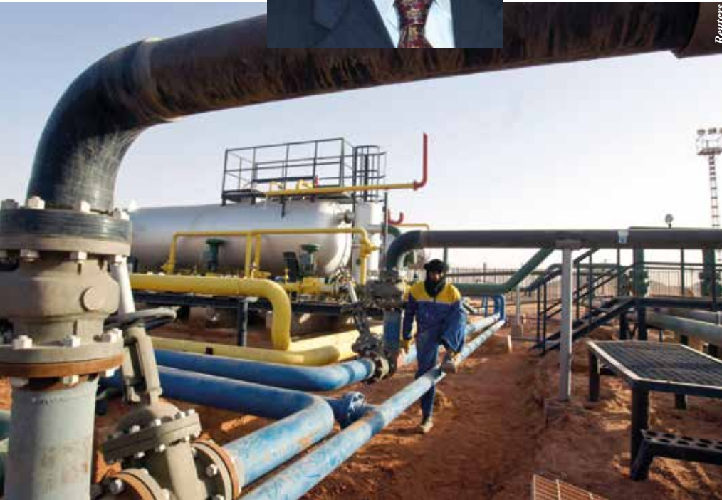
Below: A worker is seen at the Zarzaitine gas field in In Amenas, 1,600 km south-east of Algiers.
