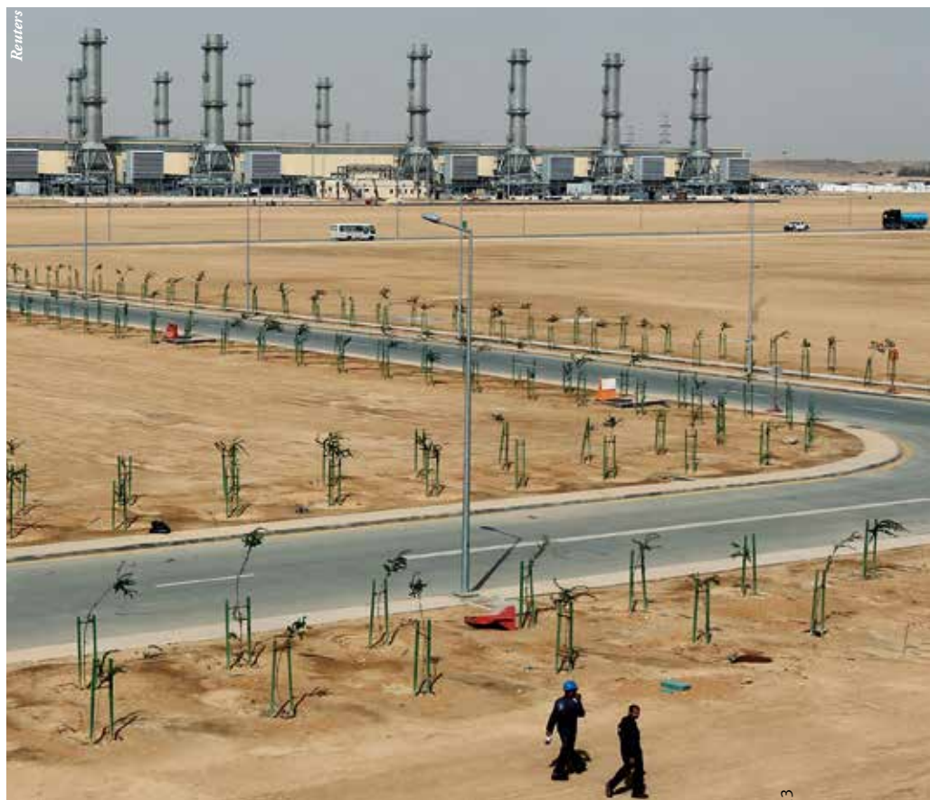
Power plant number 10 at the Saudi Electricity Company’s Central Operation Area, south of Riyadh.
