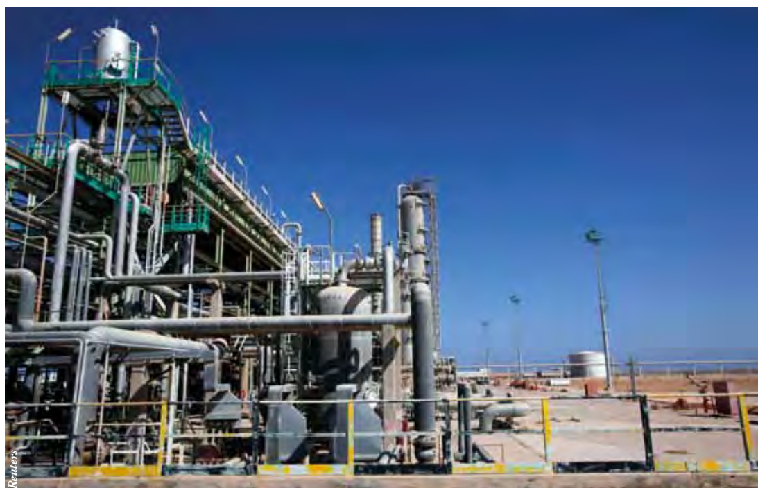
The Ras Lanuf refinery.
