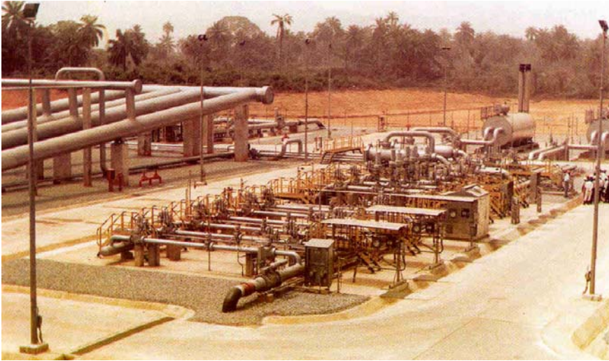
Above: Cross-section of the plant area at the Nigerian Gas Company terminal station in Ikot Abasi where natural gas is being supplied to the Aluminum Smelter Company of Nigeria
